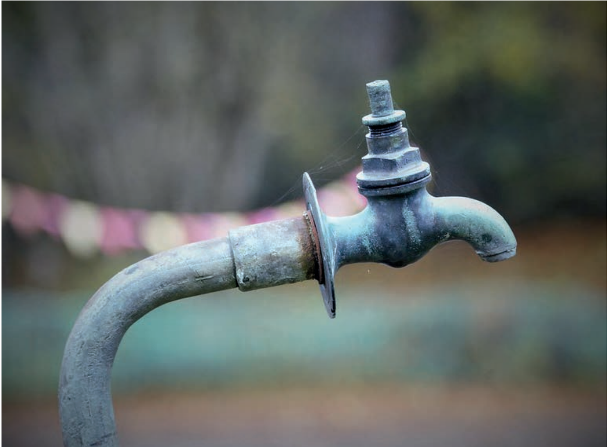
Figure 53: Non-functional water tap (© Jason Allardyce)
