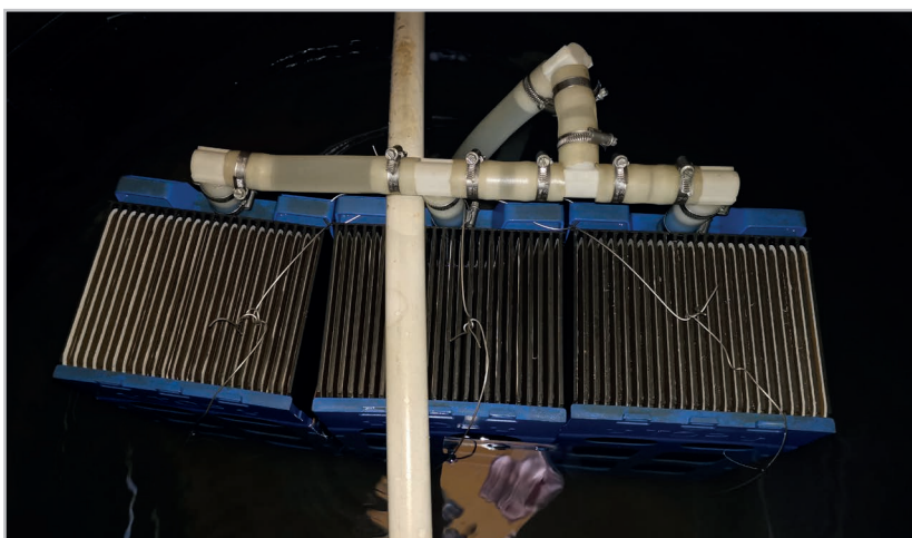
Figure 45: Three TDS-MC-MCXS2 membrane modules installed in Liberia
