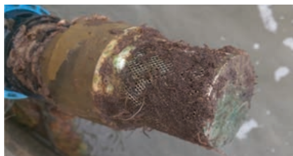
Figure 14: Clogged strainer due to lacking maintenance
