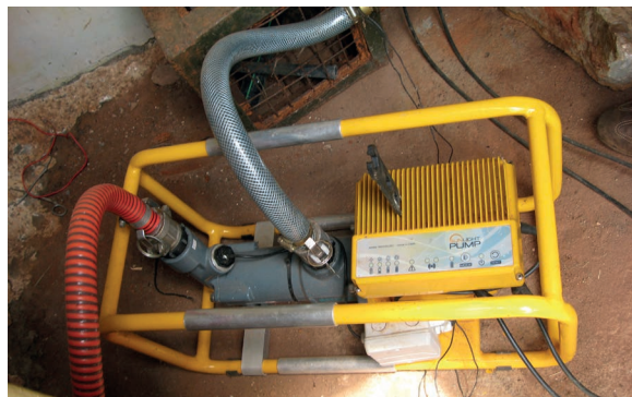
Figure 20: Ennos Sunlight pump installation
