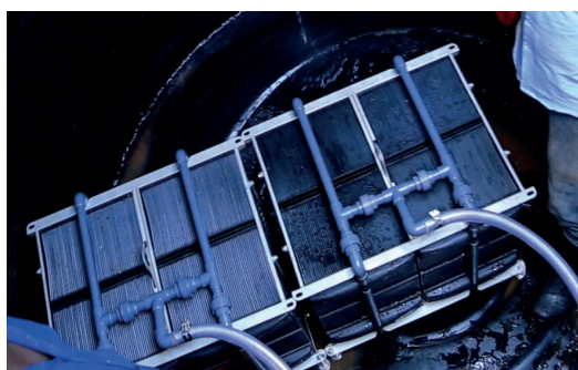
Figure 26: Aqua Cube modules in the membrane tank
